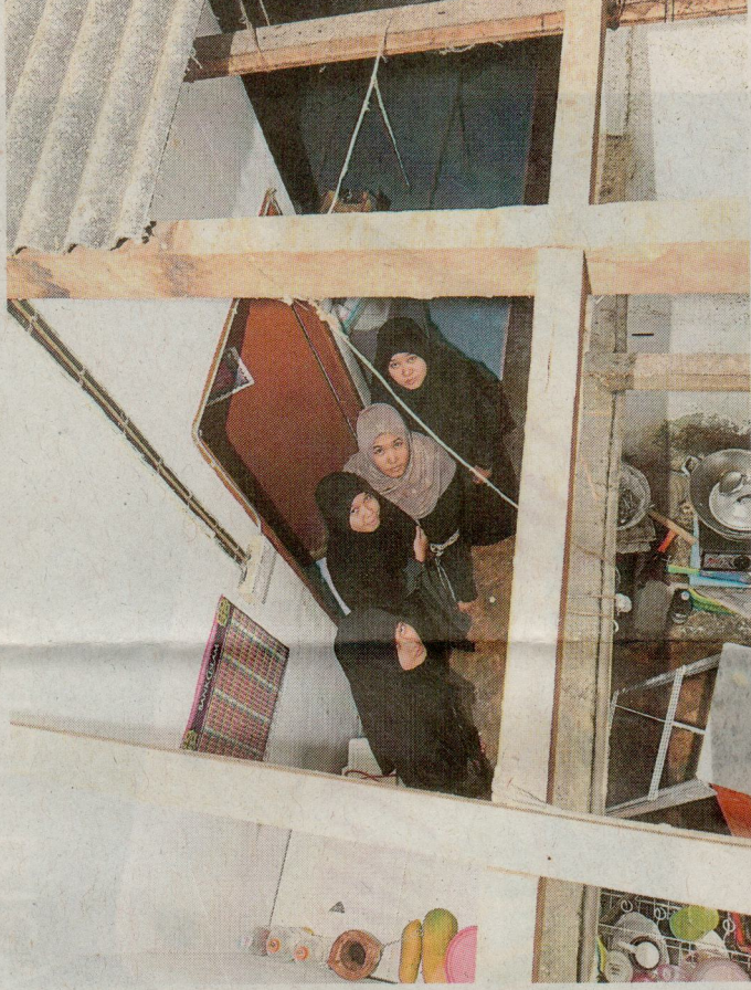
The aftermath: Kuin students checking the extent of the damage caused by the strong winds on their rented house in Taman Wira Mergong in Alor Setar, Kedah.
